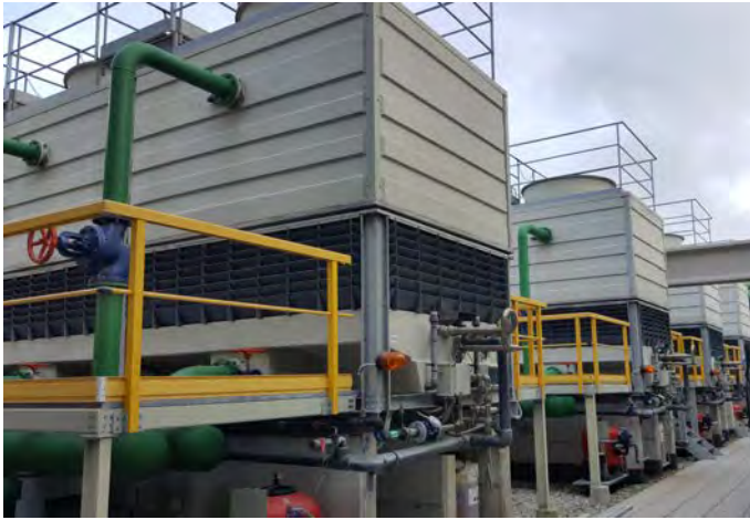
Rubí Plant (Barcelona) 4 towers of 2,500 KW each Total: 10MW
