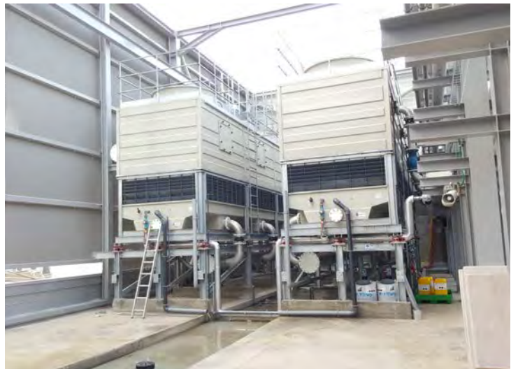
2 towers of 4,600 KW each Total: 9.2 MW
