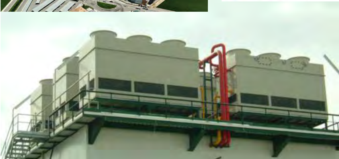
Mollerussa (Lleida) 6 NH 3 evaporative condensers Total: 8.4 MW
